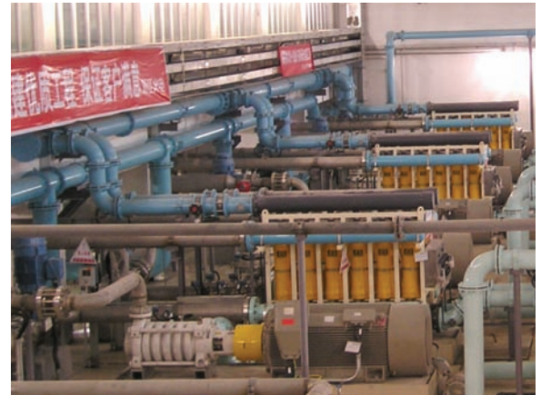
YuHuan Power Plant, China — Process Room
