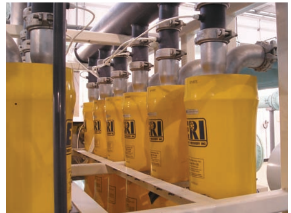
YuHuan Power Plant, China — Trains #1 and #2
